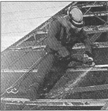
Fig 4.20: Grinding off the old welds after a section of panel had been removed. (Photograph by courtesy of University of Manchester Archives)
